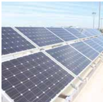
The photovoltaic system on the warehouse roof.
